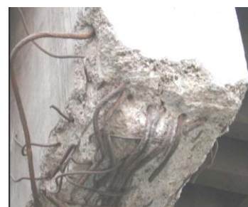
Fig. 4: Girder with exposed reinforcement
