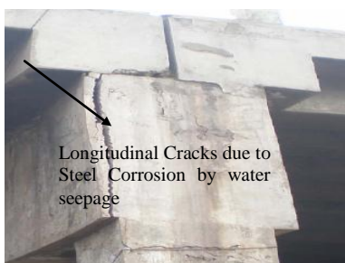
Fig. 2: Bridge girder having sewer deterioration
