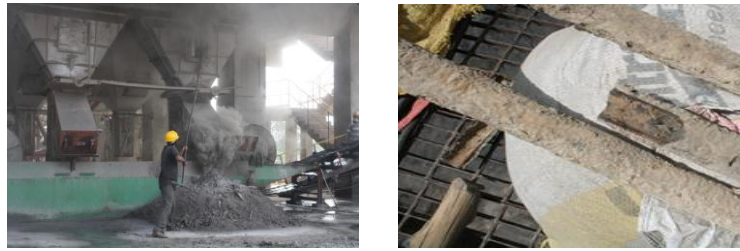
Fig. 2: Manual ash clogging removal (left) and super heater corrosion (right) [14].
