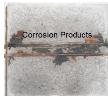
Fig. 4. Photograph of upper concrete surface and wires
