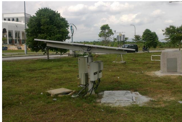
Fig. 1: Field setup of 1 kW Fixed Flat (FF) PV Generator system. Courtesy of Sichuan Zhonghan Solar Power Co. Ltd.
